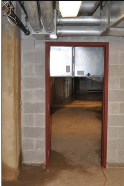
*Picture 7 - Basement door partially obstructed by duct work, taken February 23, 2011.
