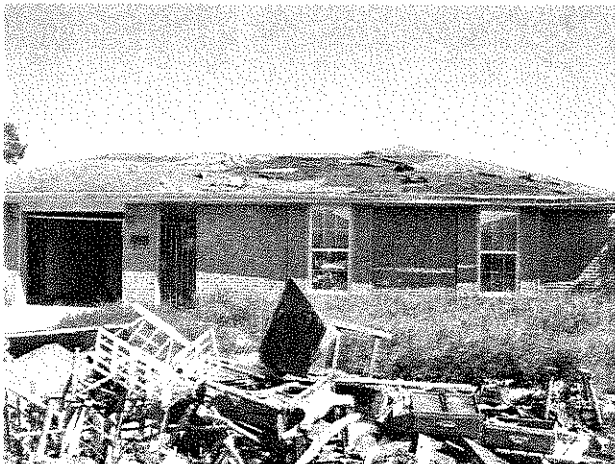
Figure 7: Brick-veneered house in Chalmette, LA after recession of 8-9 feet of flood water.
